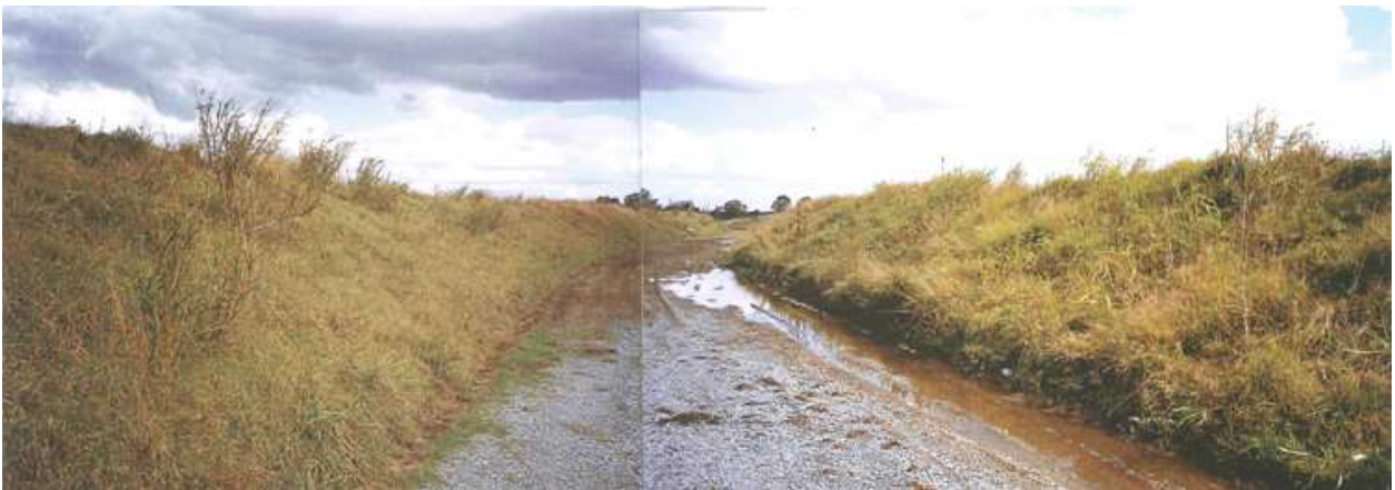
Figure 2 - The road as it existed prior to privatisation and before the first significant rain event which caused extensive scouring and environmental degradation widening and deepening it further. Attempts were made to reduce this degradation by slowing water flows. The only viable solution was to engineer an expensive drainage system which now resides below the sealed road. This road has opened up areas to the West of the airport helping fund the necessary drainage works.
