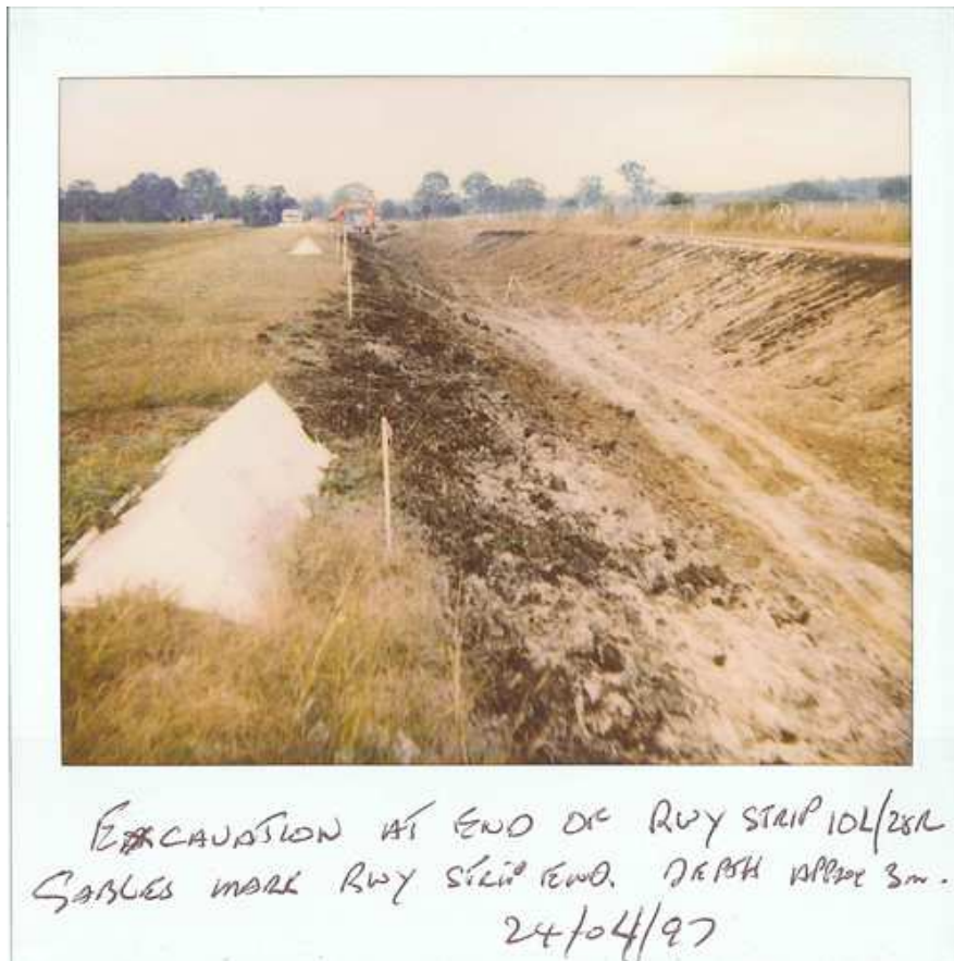
Figure 1 - "Excavation at end of Runway Strip 10L/28R. Gables mark Runway Strip end. Depth Approx 3m. 24/04/97"
